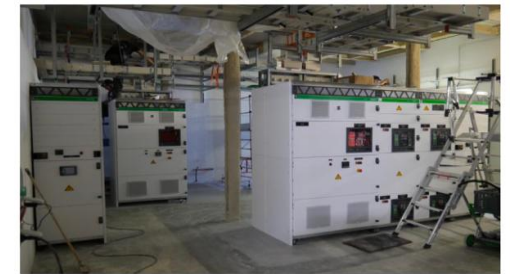
low voltage switchboard
