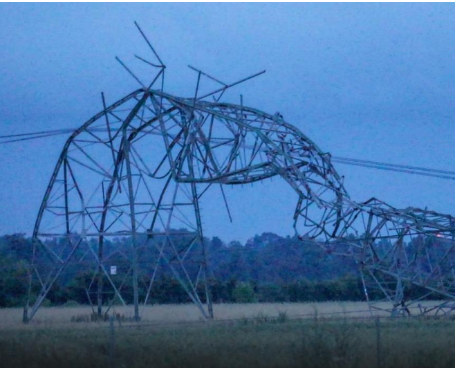
Damage of poles
