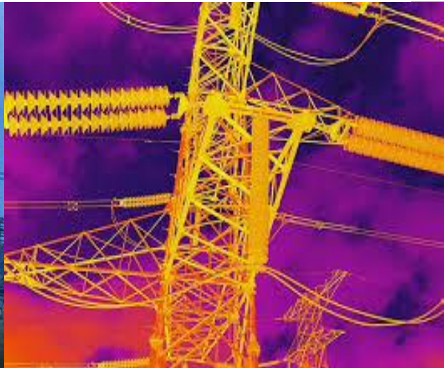
Overheating of cables/ transformer efficiency loss
